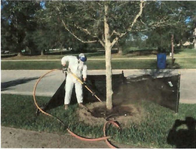
Image 4 When many trees should have a root crown excavation, a pneumatic excavation device called an Air Spade or Air Knife is used to remove soil from the root crown without damaging or otherwise wounding the roots. (Photo taken in Jacksonville)
