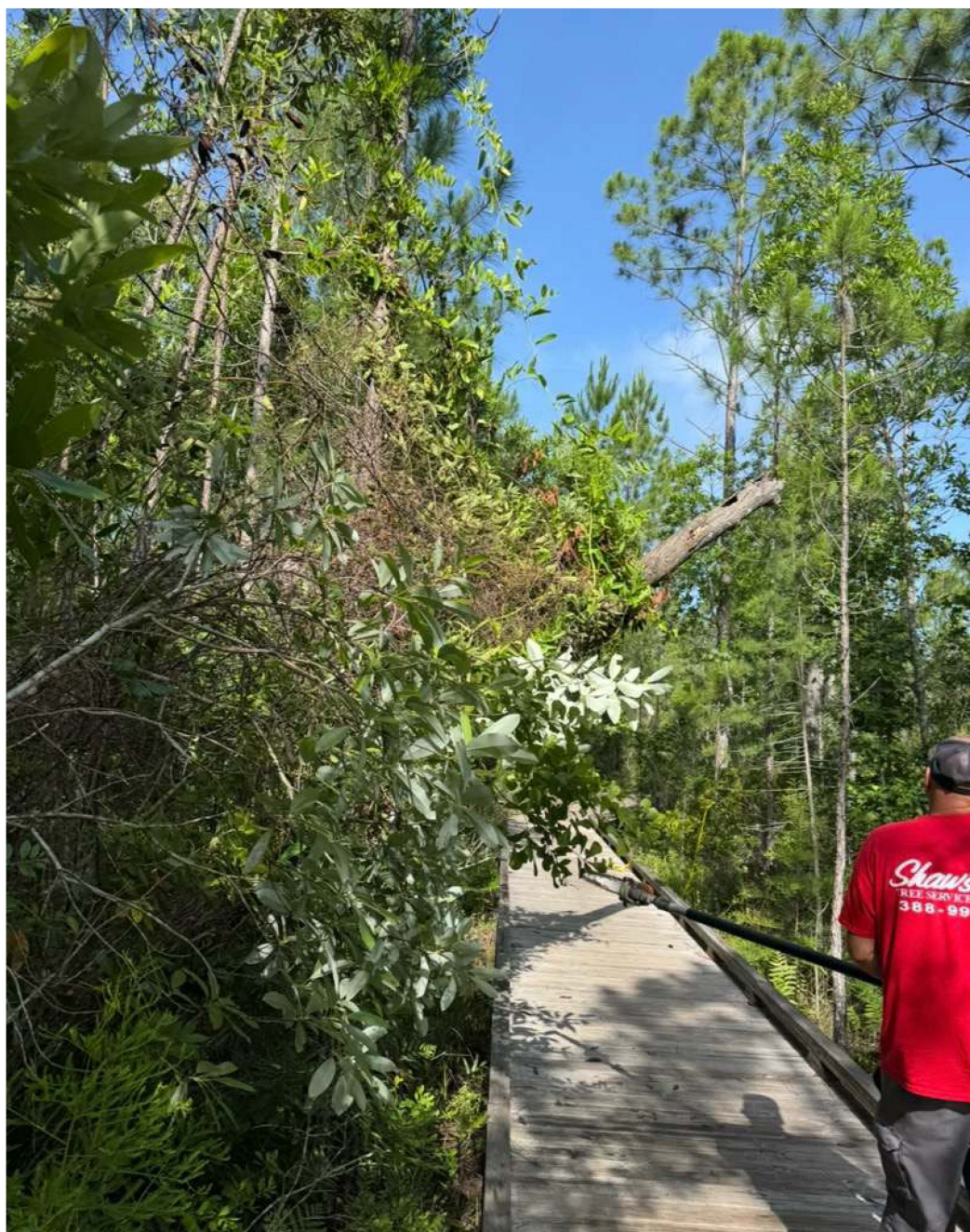
Removed Downed Tree Over Boardwalk
